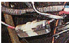
Hidden fuse revealed
